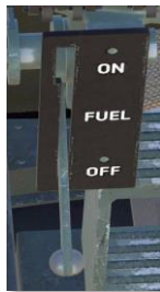
Figure 82: Main fuel valve
