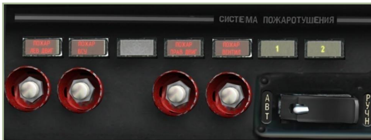
10-19: Fire extinguishing system control panel
